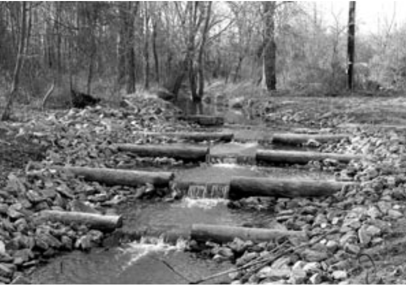
Fish Ladder at Maydale Nature Center
