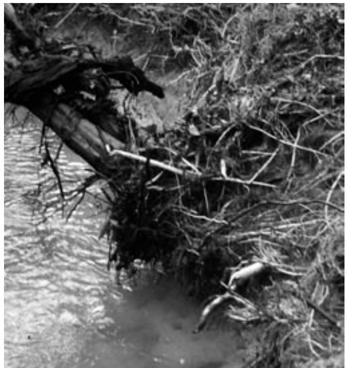
Freshly exposed roots in this streambank on the Good Hope tributary are irrefutable evidence of significant erosion.
